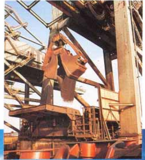
Bulk handling hoppers and chutes.
