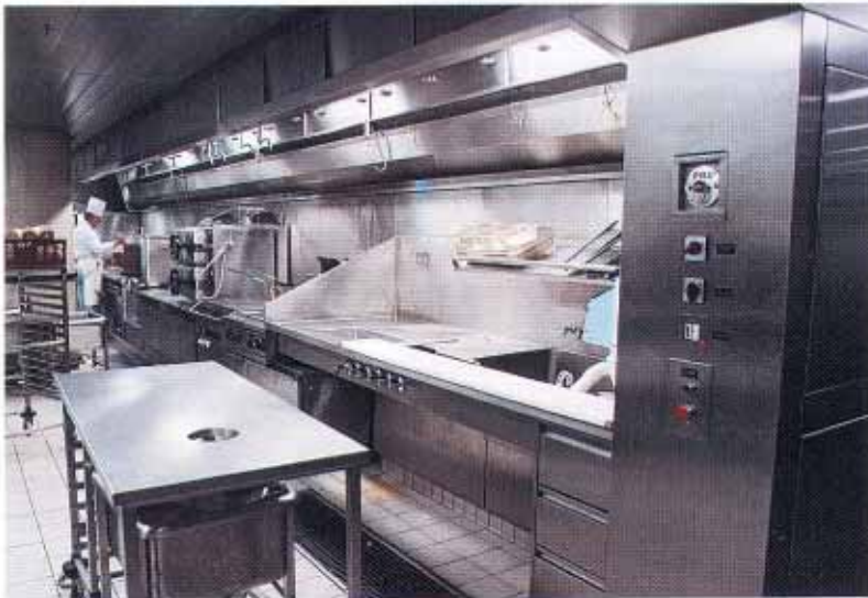
Commercial catering equipment.
